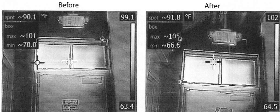
Figure 2: Window above the door shows an increase in the internal temperature of the building, signifying better insulation. This is the work of one of the student groups with a community partner.
